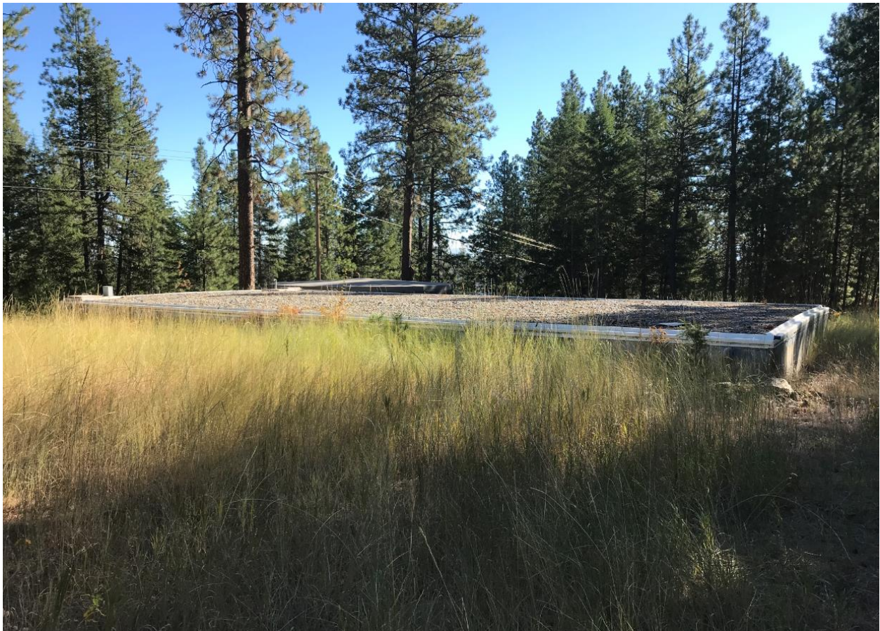
Figure 5: Greensferry Water District reservoirs, recently approved for a new booster pump to accommodate increasing demand
